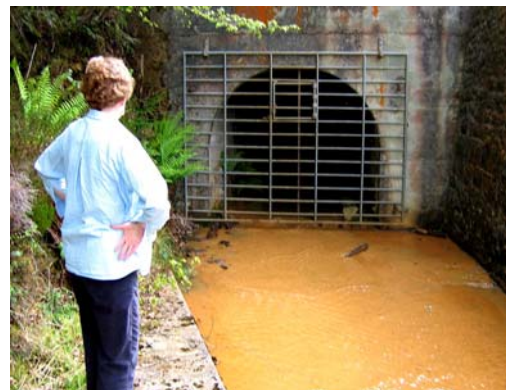
Parc Lead Mine in the Gwydyr Forest will be on the initial list of NRW sites in the agreement pioneered by Elsie Little
